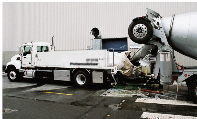
Fig. 4.4.1—Truck-mounted city pump.
